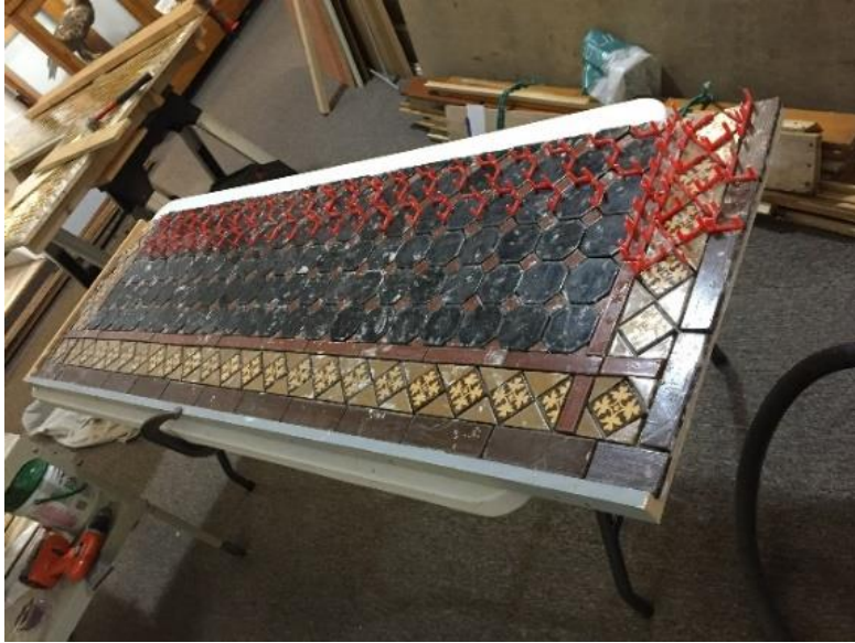
Hearth tiles placed on plywood prior to grouting. Note the red plastic spacers between some tiles.
