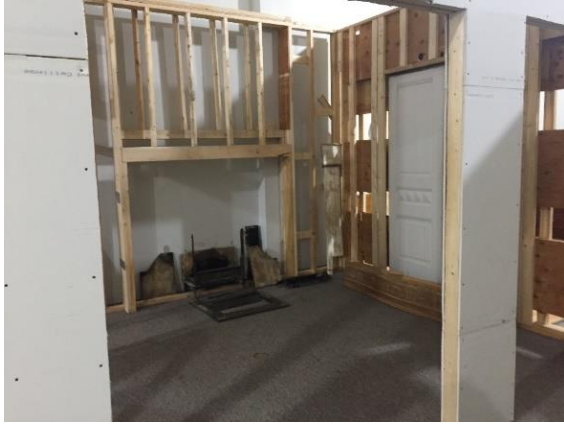
The supports for the fireplace mantel and overmantel with the fireplace insert shown in pieces.
